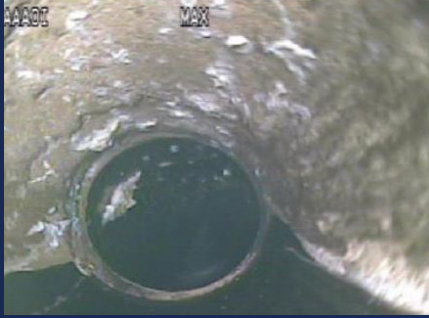
Extreme scale buildup in vacuum line
